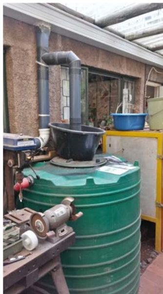
Figure 47. Rainwater harvesting from gutter into collection tank (Author, 2014).
