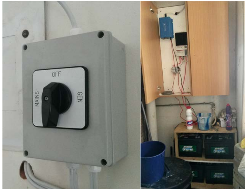
Figure 32. Supply switch and battery store (Author, 2014).
