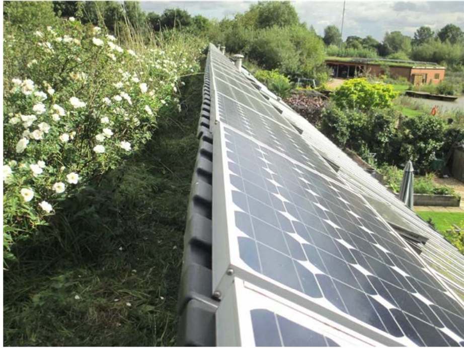
Figure 29. Photovoltaic array on roof (Alasdair Morrison and Partners).
