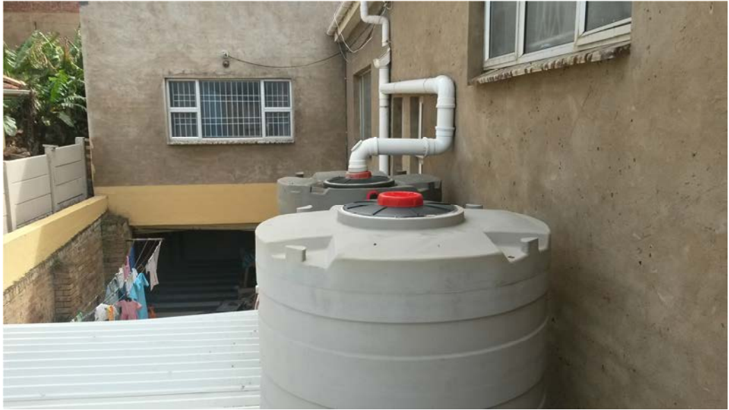
Figure 33. Rainwater harvesting collection tanks (Author, 2014).
