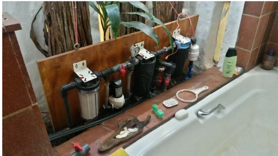
Figure 48. Rainwater filtration system (Author, 2014).
