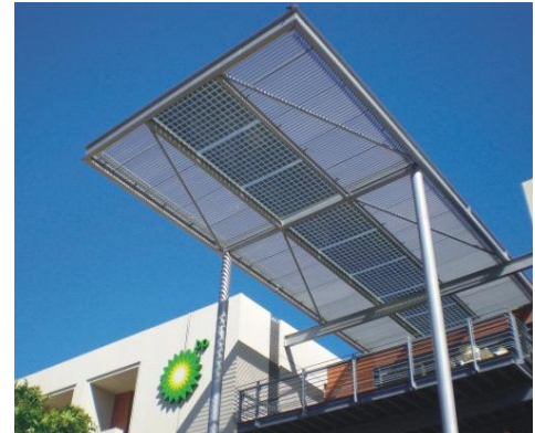
Fig. 5.5.2- Photograph of the PV panels at the entrance to the BP Head Offices (Source- By Author)
