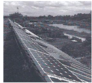
Fig. 4.2.21- Photograph of the 7,6 kW photovoltaic array (Source- Sassi: 2006, 45)
