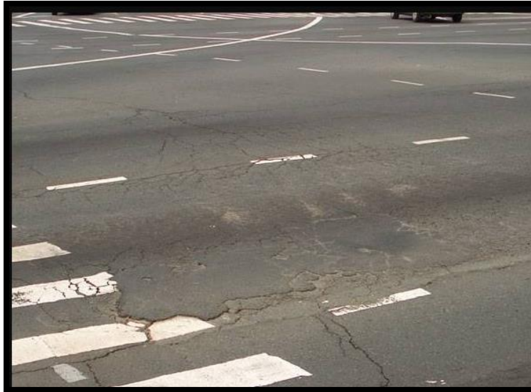
Figure 2.6: Image indicating crocodile cracks
