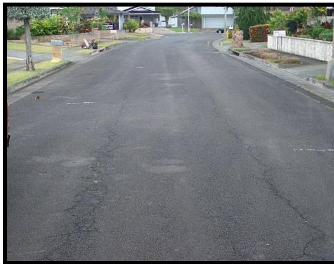
Figure 2.7: Image indicating Longitudinal Cracks
