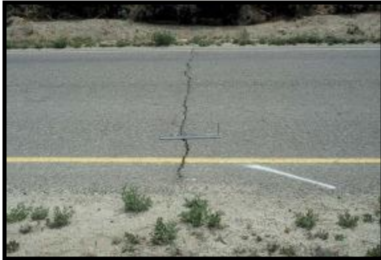
Figure 2.8: Image indicating Transverse Cracks
