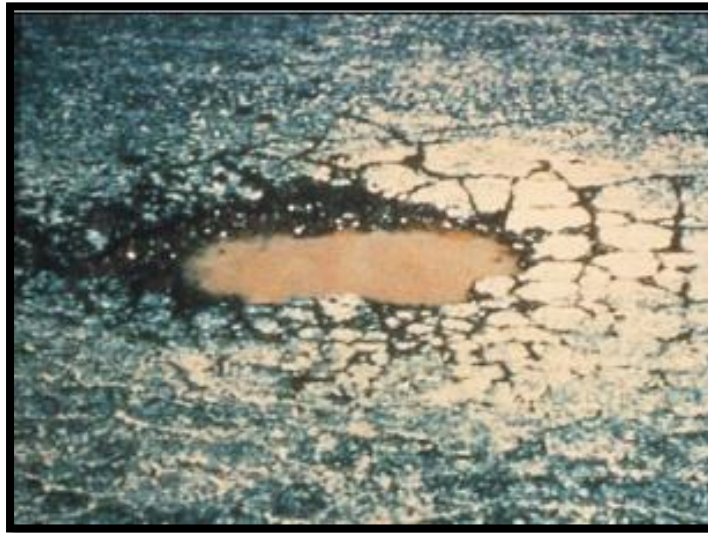
Figure 2.10: Image indicating a severe pothole
