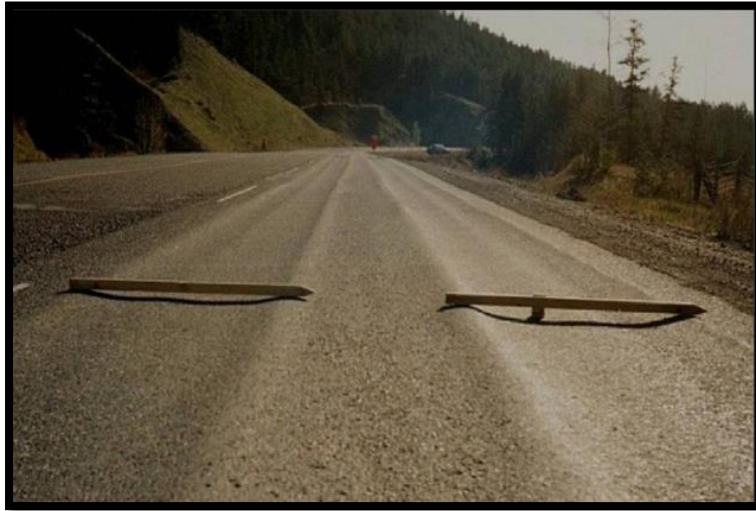
Figure 2.11: Image indicating severe Rutting of road below straight edge
