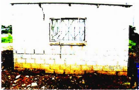
Figure 7 : Structural crack starting from roof.
