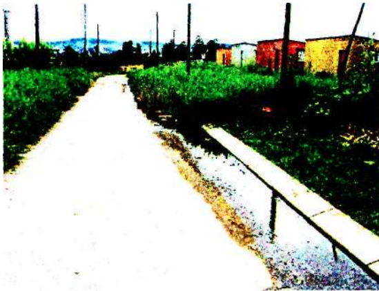
Figure 15 : Poor service maintenance.
