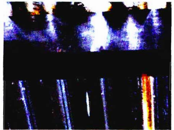
Figure 10: Poor sealing of holes, as is evident from reflection of light on the beam.
