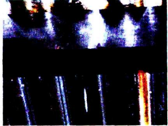
Figure 10: Poor sealing of holes, as is evident from reflection of light on the beam.
