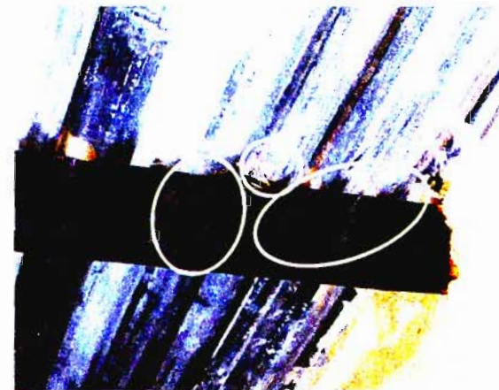
Figure 12: Poor material (knotty timber), nailing roof screws, poor and holes not sealed.
