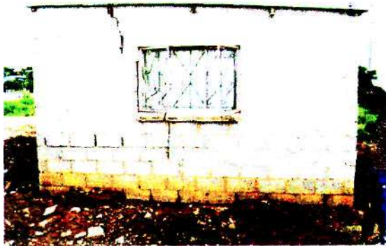
Figure 7 : Structural crack starting from roof.
