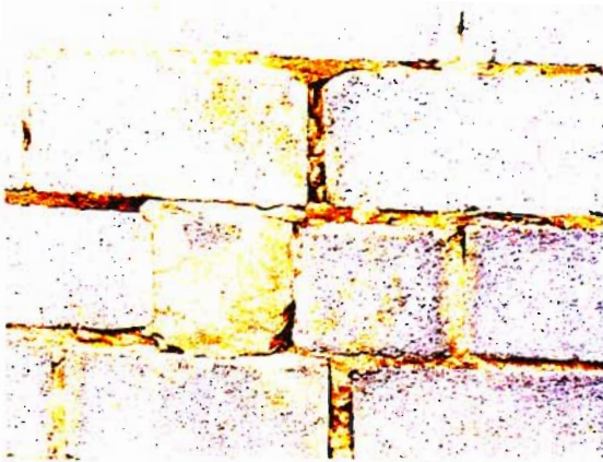
Figure 1 : Poor mortar mix, inadequate cement.
