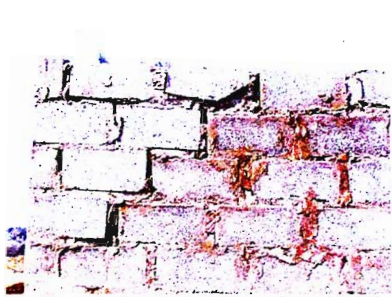
Figure 2 : Poor block work resulting in re-work.
