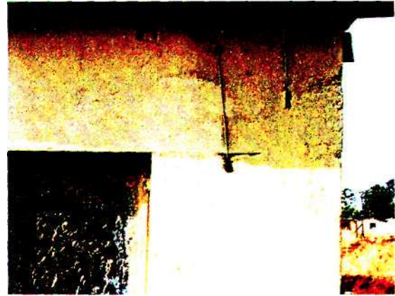
Figure 14 : Poor beam filling, roof ties fitted retrospectively, and holes not sealed.
