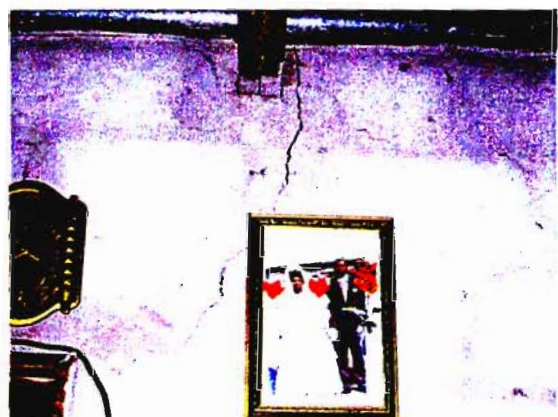
Figure 6 : Structural cracks from roof beam to window.
