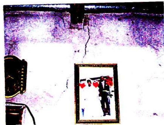
Figure 6 : Structural cracks from roof beam to window.
