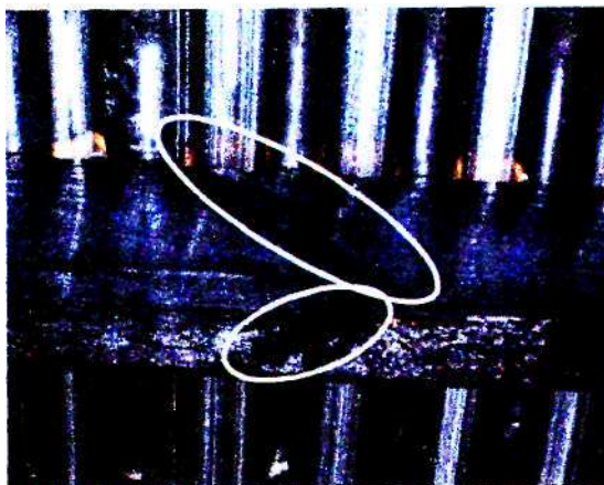
Figure 11 : Poor quality timber used.
