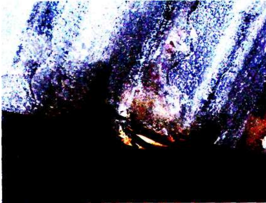
Figure 9: Roof screw not done properly.
