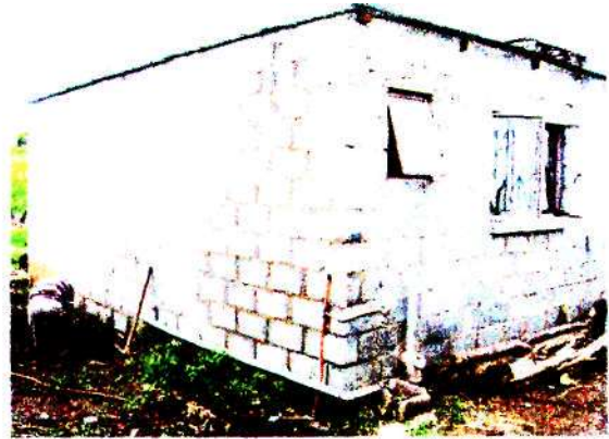
Figure 8 : Foundations being underpinned as a result of poor founding. Also note block-work had to be redone.
