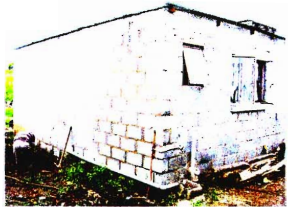
Figure 8 : Foundations being underpinned as a result of poor founding. Also note block-work had to be redone.
