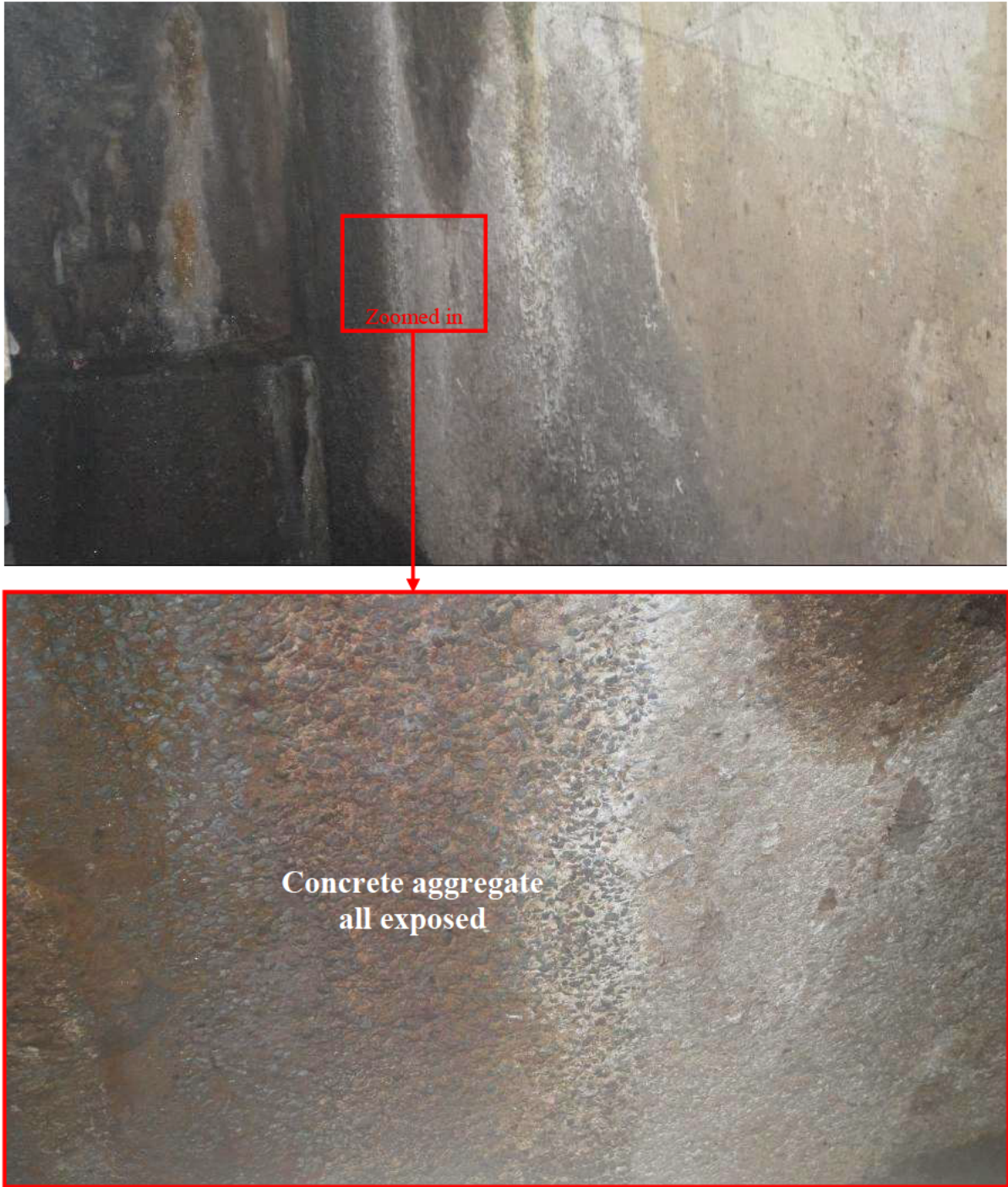
Figure 4-3: Corroded concrete wall
