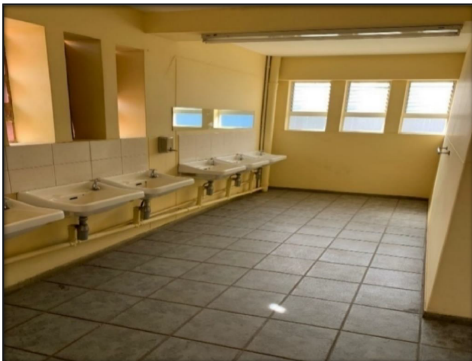
Figure 6.41. College C: Female Ablution Facilities—Hand Washing Sinks
