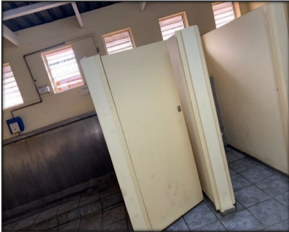
Figure 6.43. College C: Ablution Facilities Male Urinal and Toilet Stall
