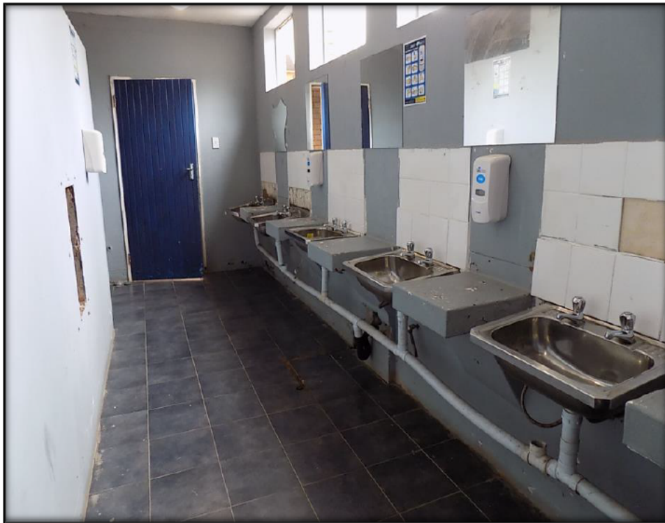
Figure 6.9. College A: Ablution Facilities—Handwashing Sinks
