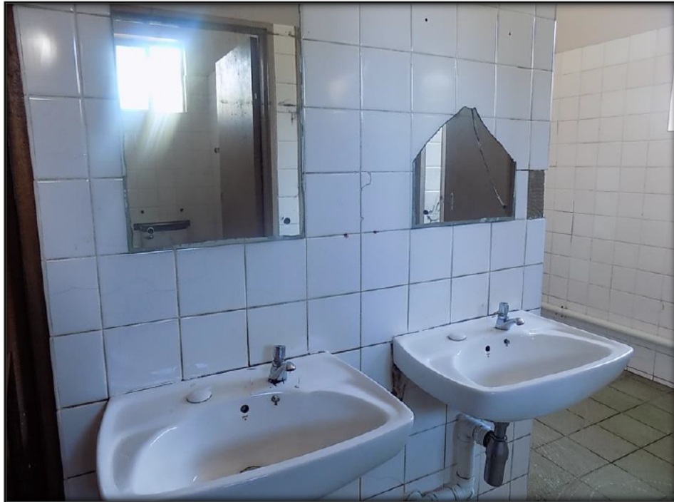
Figure 6.30. College B: Ablution Facilities—Hand Washing Sinks
