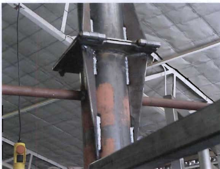
Figure 3.10 Crane hinge point with the support girders and handles.
