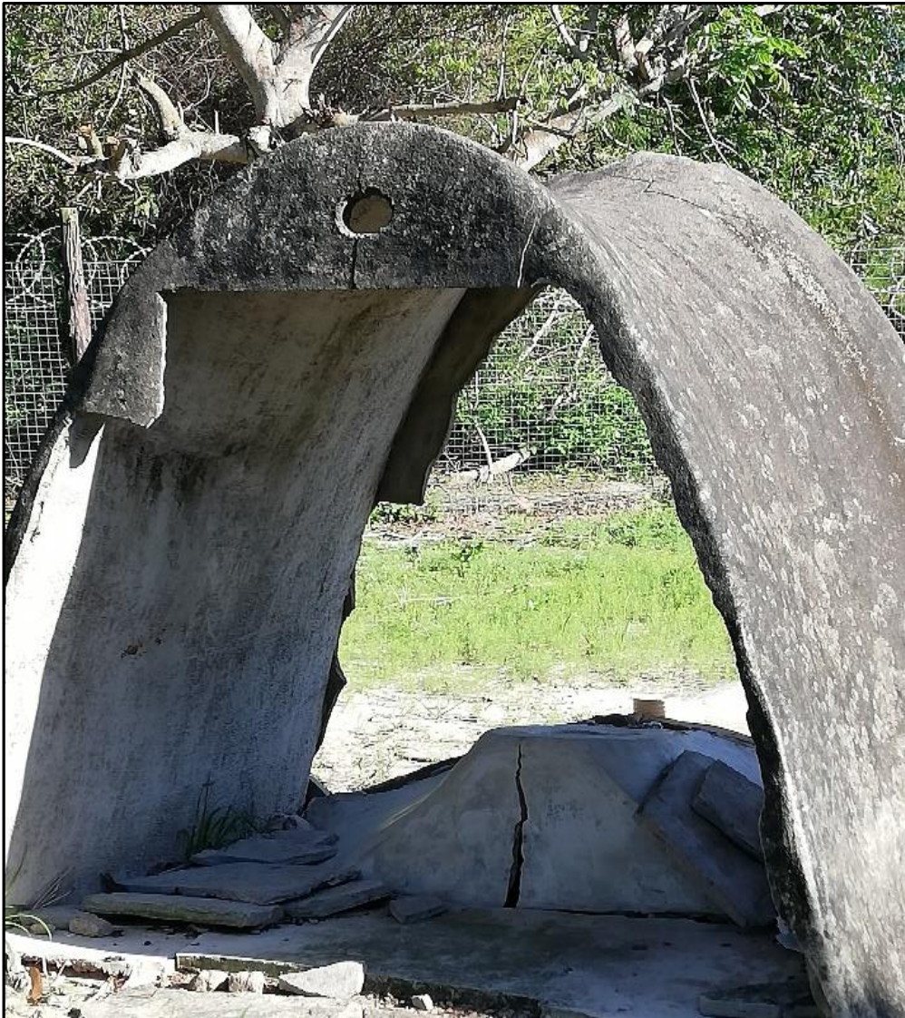
Figure 0.7. The disrepair of a pit latrine installed 2010 in Ward 11, uMhlabuyalingana LM
