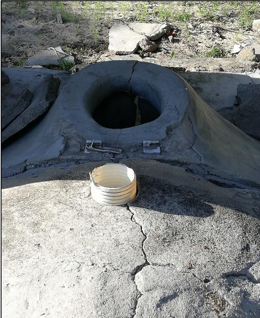
Figure 0.8. The disrepair of a pit latrine installed 2010 in Ward 11, uMhlabuyalingana LM
