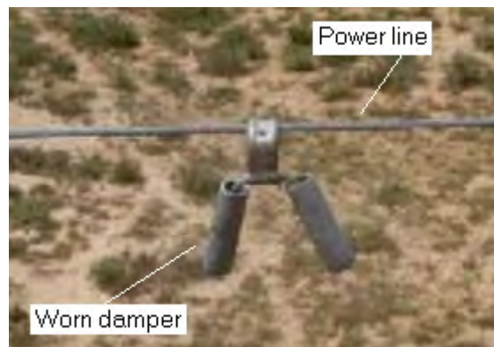
Figure 3.4: Photograph of a worn Stockbridge damper on a power line (Retief, No Date).
