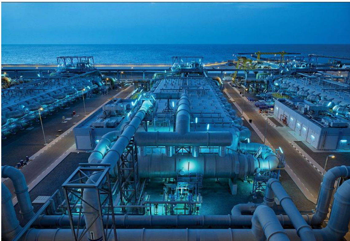
Figure 2.2: Desalination plant in Dubai (Kelsey, 2017).
