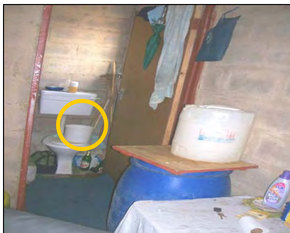
Figure 4: A toilet in Old Dunbar which is not flushable highlighted by a yellow circle.
