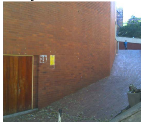
Plate 6.3 The blank facade is described as the ‘back’ of the building (Authors own image)
