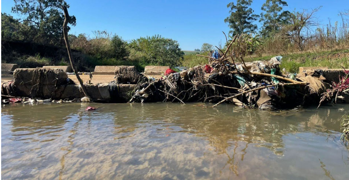
Supplementary information Figure S3.5: The slimy floor from sewage and industrial pollution at lower Baynesspruit and uncollected or illegal dump refuse clogging the culvert.
