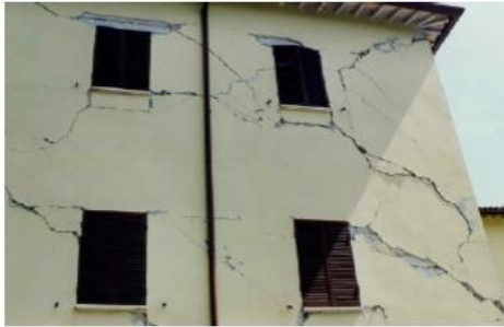
Figure 8: Building damage due to in-plane loading.
