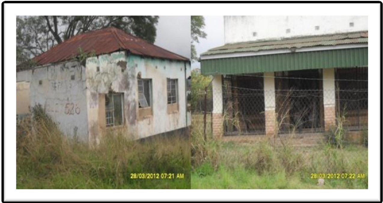
Figure 5.6 Abandoned (dilapidated) houses along the Edendale stadium node corridor section
