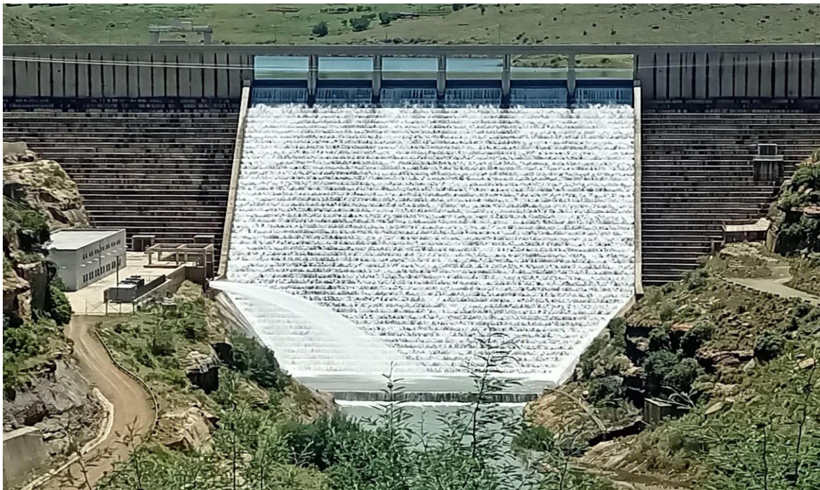
Figure 3.5 Metolong Dam at full supply level releasing floodwaters through its ogee spillway on 25 December 2020. The controlled discharge highlights the dam’s operational role in attenuating peak flows and regulating downstream hydrology within the South Phuthiatsana Catchment.
