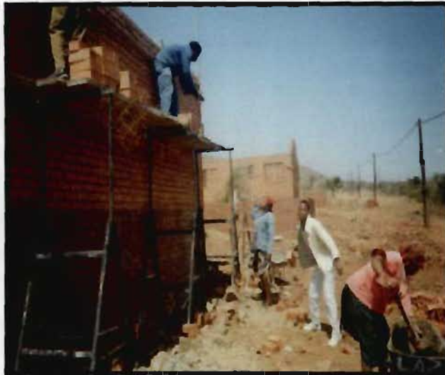
NB The man in a white suit is a clerk of works and not a labourer
