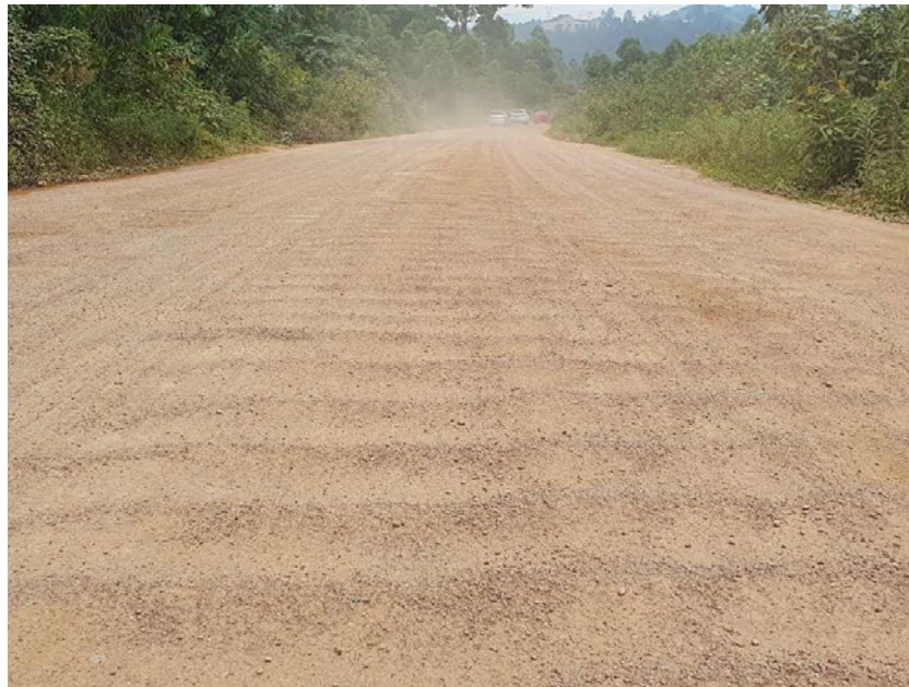
Plate 4-1: Section of Ingweni road in Pinetown, SA showing corrugation failures
