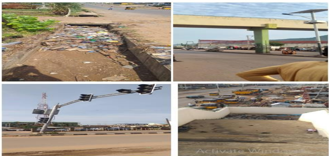
Figure 7.20: Road and Road Fixture Conditions in Lokoja
