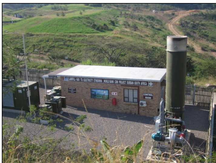
Figure 8: Gas-to-electricity plant at Mariannhill Landfill Site
