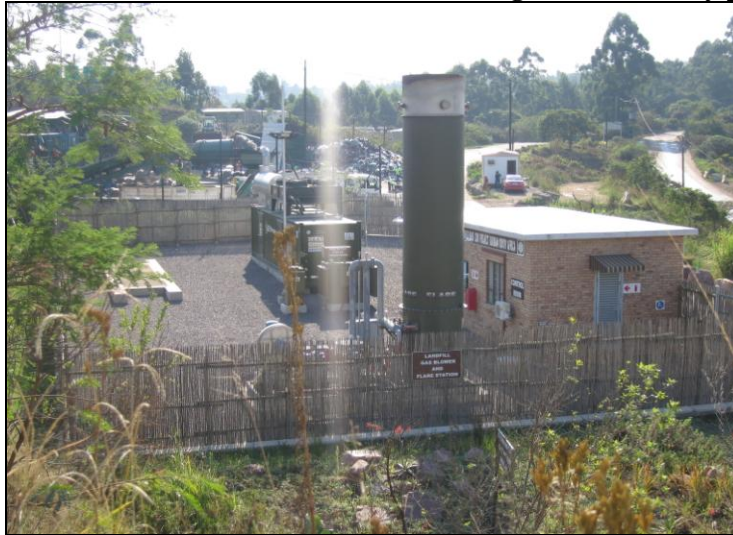
Figure 9: Gas blower and flare station section of the gas-to-electricity project
