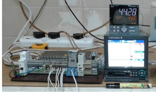
Figure 3-9: Power supply unit
