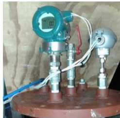
Figure 3-5: Digital pressure transmitter, thermocouple and pressure breaker valve
