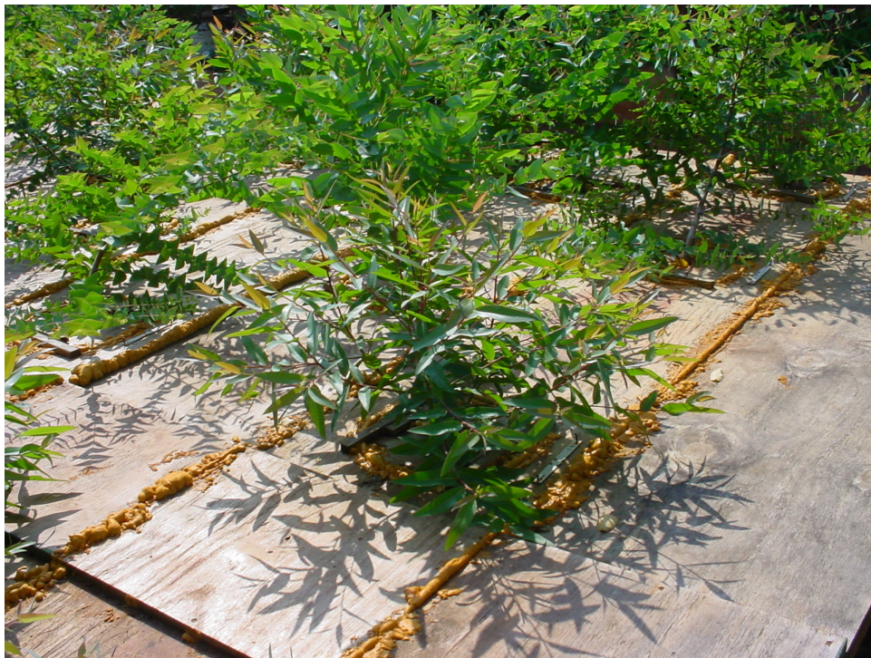
Figure 2.11: Top view of the box with one-component polyurethane foam applied where the individual shutterboard sheets met.
