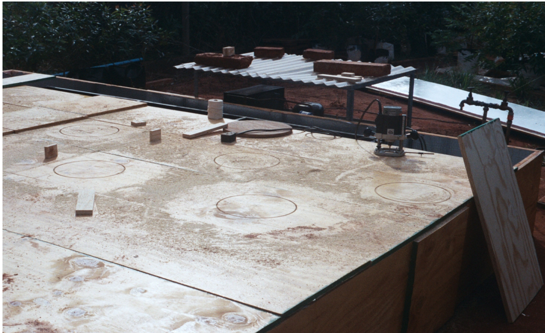
Figure 2.4: Twenty five 300 mm holes were cut in the lid to insert the 25 plants.
