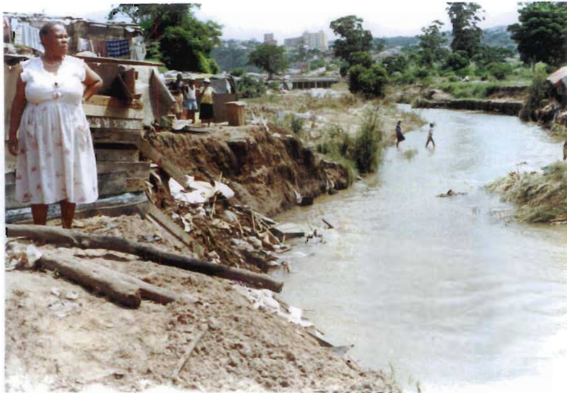
Figure 3.12 Illustration of flood damage to shacks in Quarry Road West: The stream has washed between the dwellings, removing topsoil and toilets. This is typical example of a slum built on a river's flood plain.
