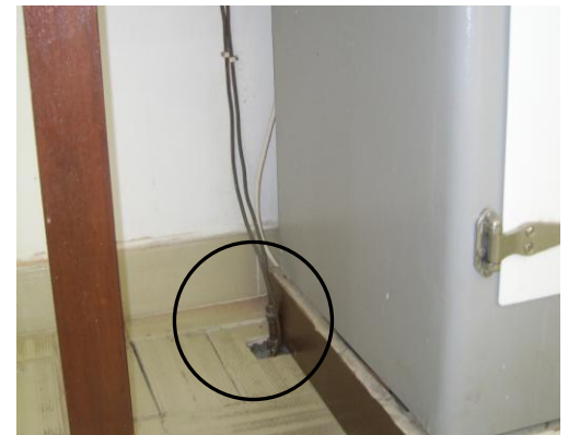
Illustration 5.3.9: pipes popping out of the floor to service laboratory equipments (Source: Author).
