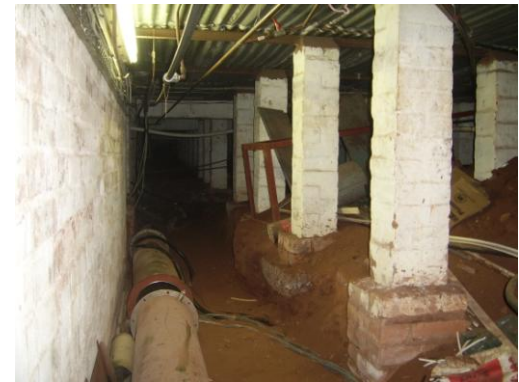
Illustration 5.3.8: the plant room in the semi basement with pipes going through the floor to service labs (Source: Author).
