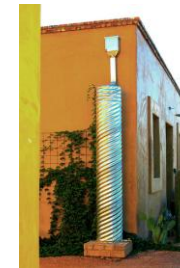
Illustration 23: Rain water collection exposed to the walkway
