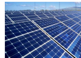
Illustration 24: Photovoltaic panels fixed on concrete slabs
