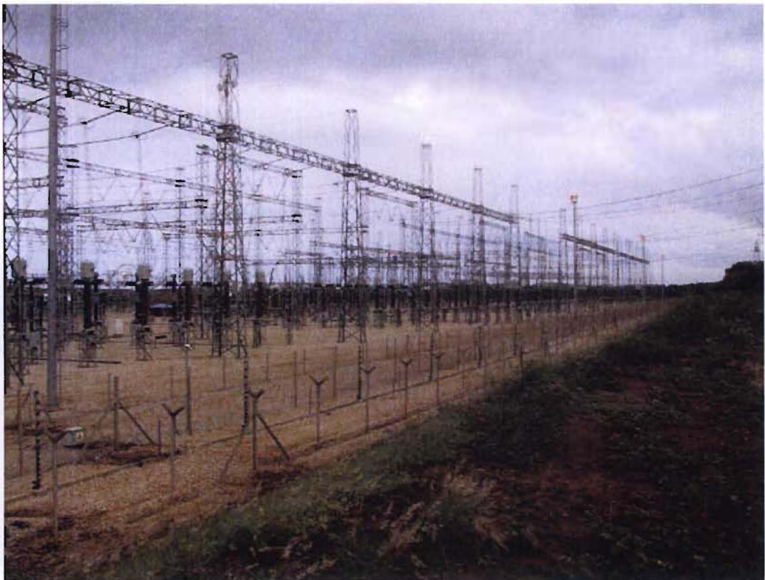
Figure 21.2: High Visual Impact Tubular Busbar Substation (Athene Substation – Empangeni - KZN)
