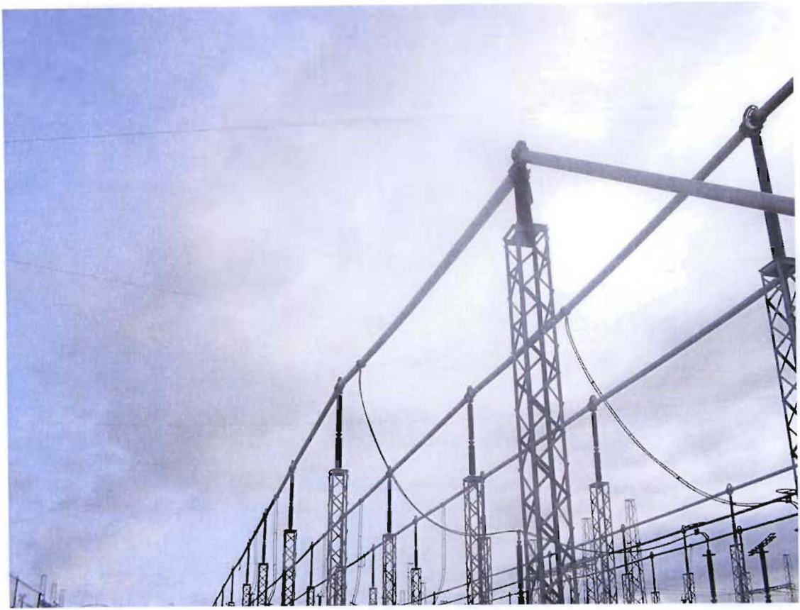
Figure 16.9: Catastrophic Failure of the 400kV Red Phase Conductors
