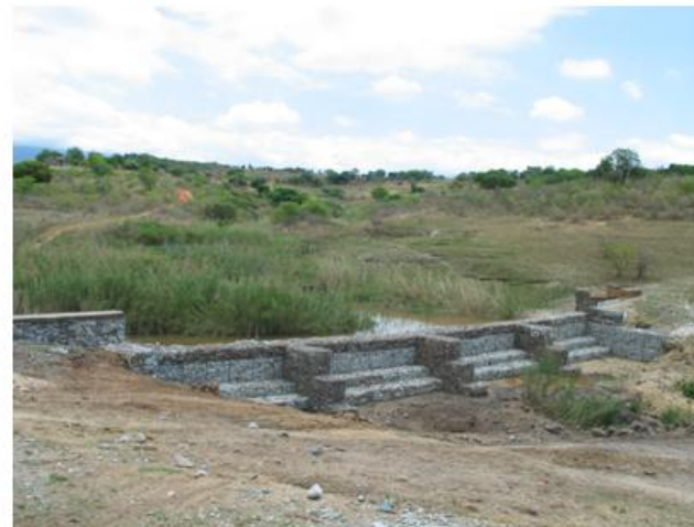
Figure 3.5: Installed buttress weir (top left, top right) with design and location of stilling well (bottom left), gabion dam (bottom right)
