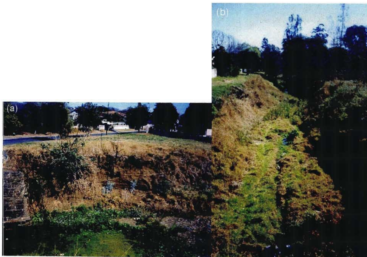
FIGURE 2: Figure 2(a) shows bank scour downstream of a bridge on the Foxhill Spruit, while 2(b) shows the incised channel form, typical of many urban streams.
