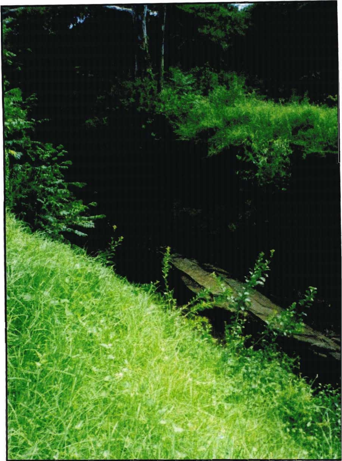
Figure 4.4: Channel incision and undercutting of outer bank with root system exposed. Foxhill Spruit, January 2002.
