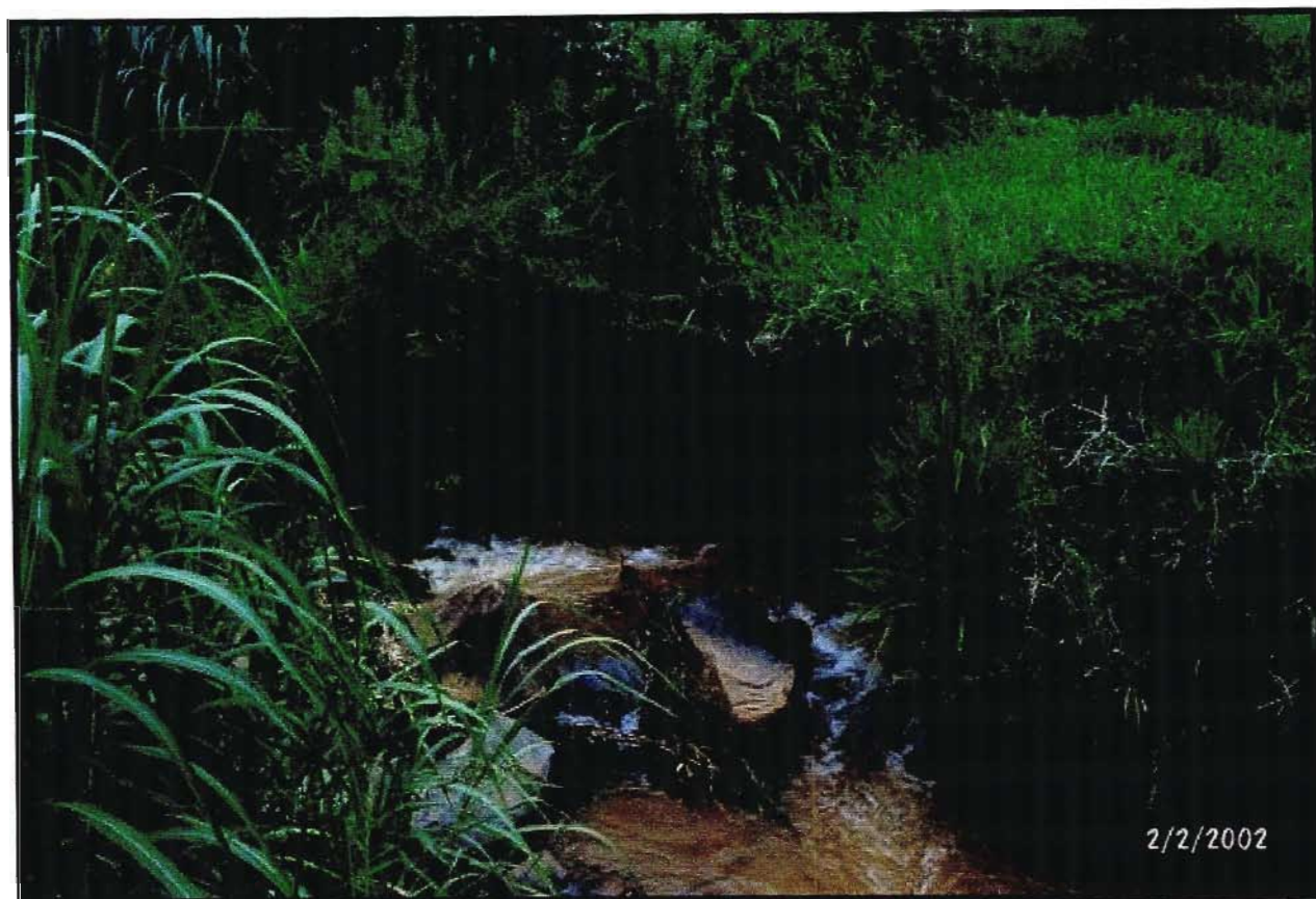
Figure 4.6: Scour of outer meander - Townbush Spruit, February 2002.
