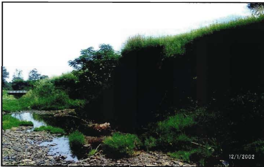
Figure 2.6: Evidence of undercutting on the banks of the Foxhill Spruit, January 2002.
