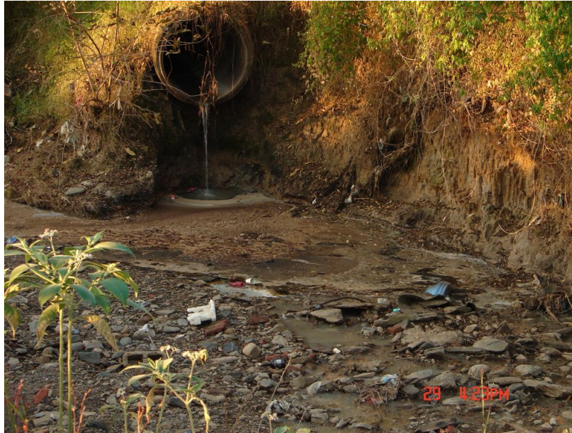
Figure 1.2: A stormwater outfall along the Baynespruit, showing pollution from both solid and liquid waste
