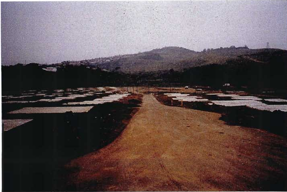
Figure 4.4. Housing and road construction on the high ground of the Mount Royal Housing Project. September 17, 2004.
