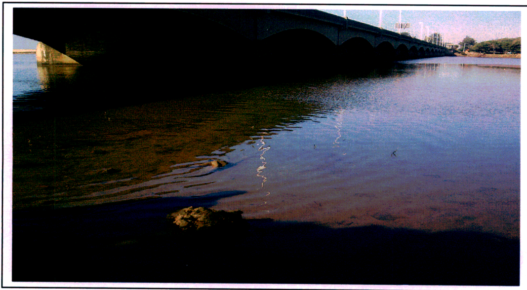
Plate 3.11 – View of the Ellis Brown Bridge constructed over the estuary. High water marks during flood events are clearly evident on the bridge walls.
