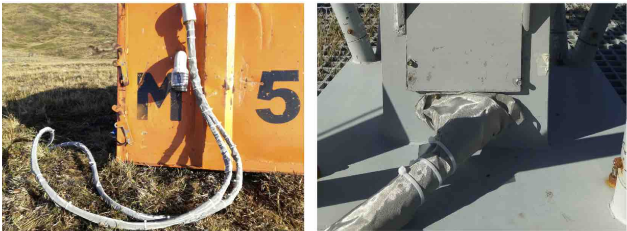
Figure 3.20: The PRI Z M cables are protected by wrapping them with finely woven steel mesh ( left ). A combination of steel mesh and scourer pads are used to prevent mice from entering the cable feeding pointing at the base of the antenna ( right ).
