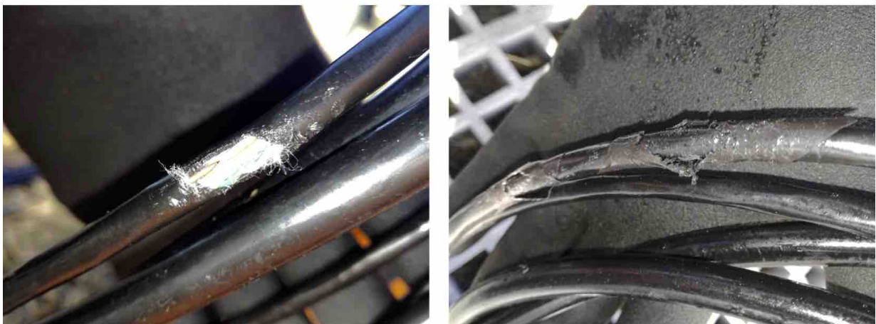
Figure 3.19: Mice eating away our cable insulation ( left ) and self amalgamating tape ( right ).
