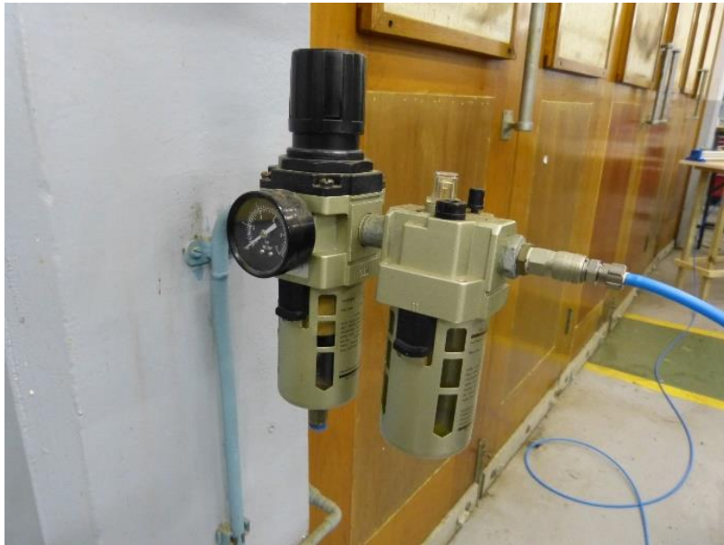
Figure 4.14: FRL service unit
