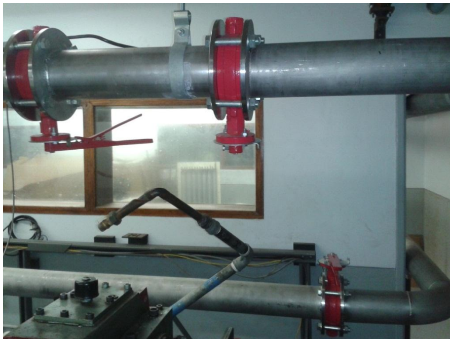
Figure 4.11: Position of the valves. The inlet valve is at the bottom and the two discharge valves at the top.
