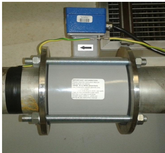
Figure 4.14: Flow meter clamped between flanges in the discharge line.
