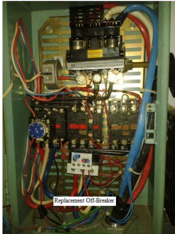
Figure 4.3: Electrical control circuitry with replacement off breaker.
