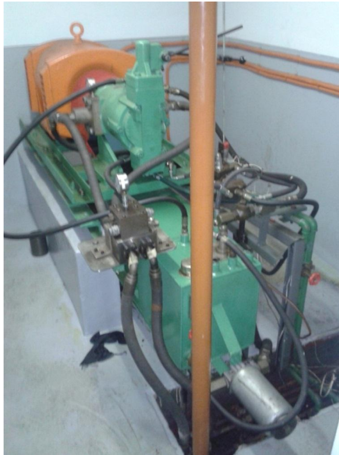
Figure 4.1: Uchida hydraulic pump and electric drive motor.
