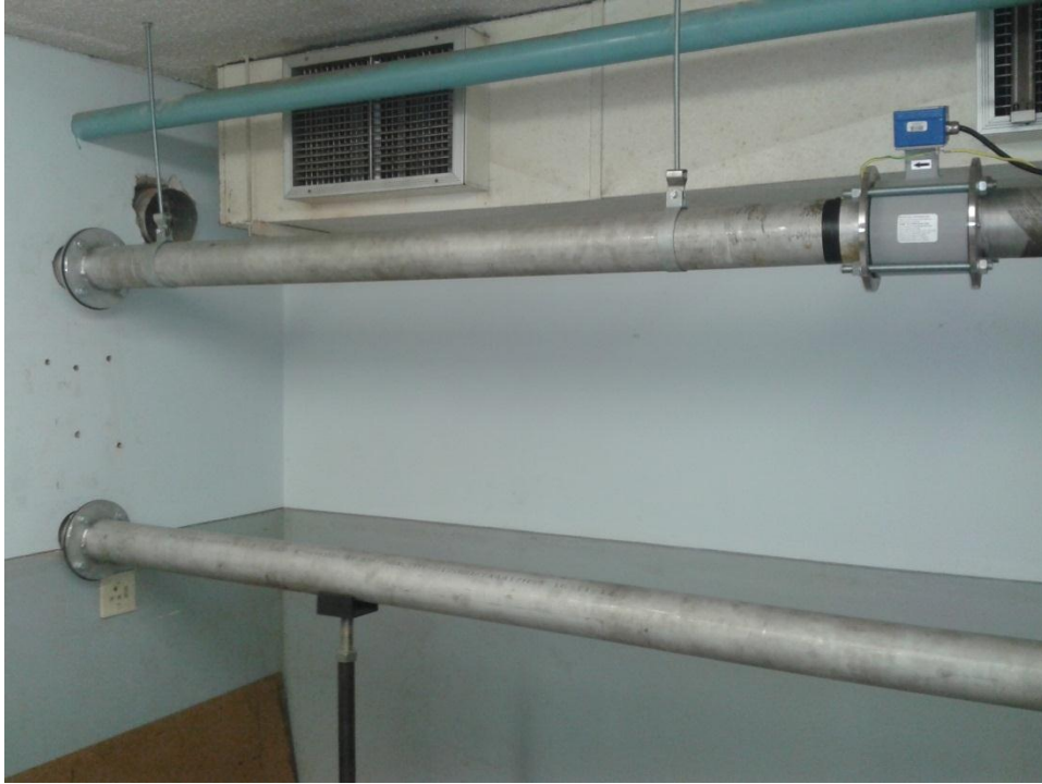
Figure 4.12: A section of the inlet and discharge piping. Holes cut through the wall can be seen on the left. Supports for the inlet line (bottom) and discharge line (top) can be seen.
