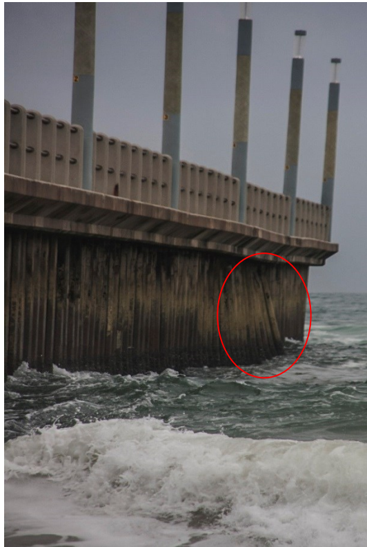
Figure 1-3: Photograph of Bay of Plenty Pier south side pile failure, highlighted in red (adapted from EMS, 2013).
