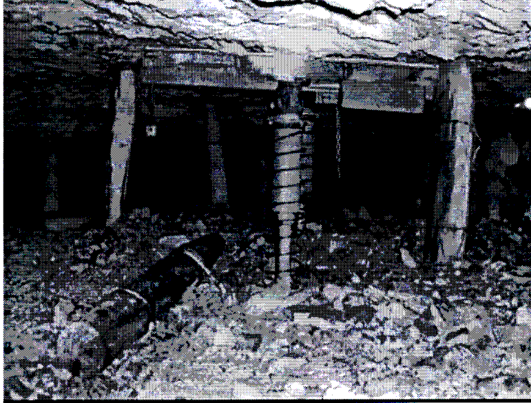
Figure 3-12 Condition of unit after being subjected to blasted rock
