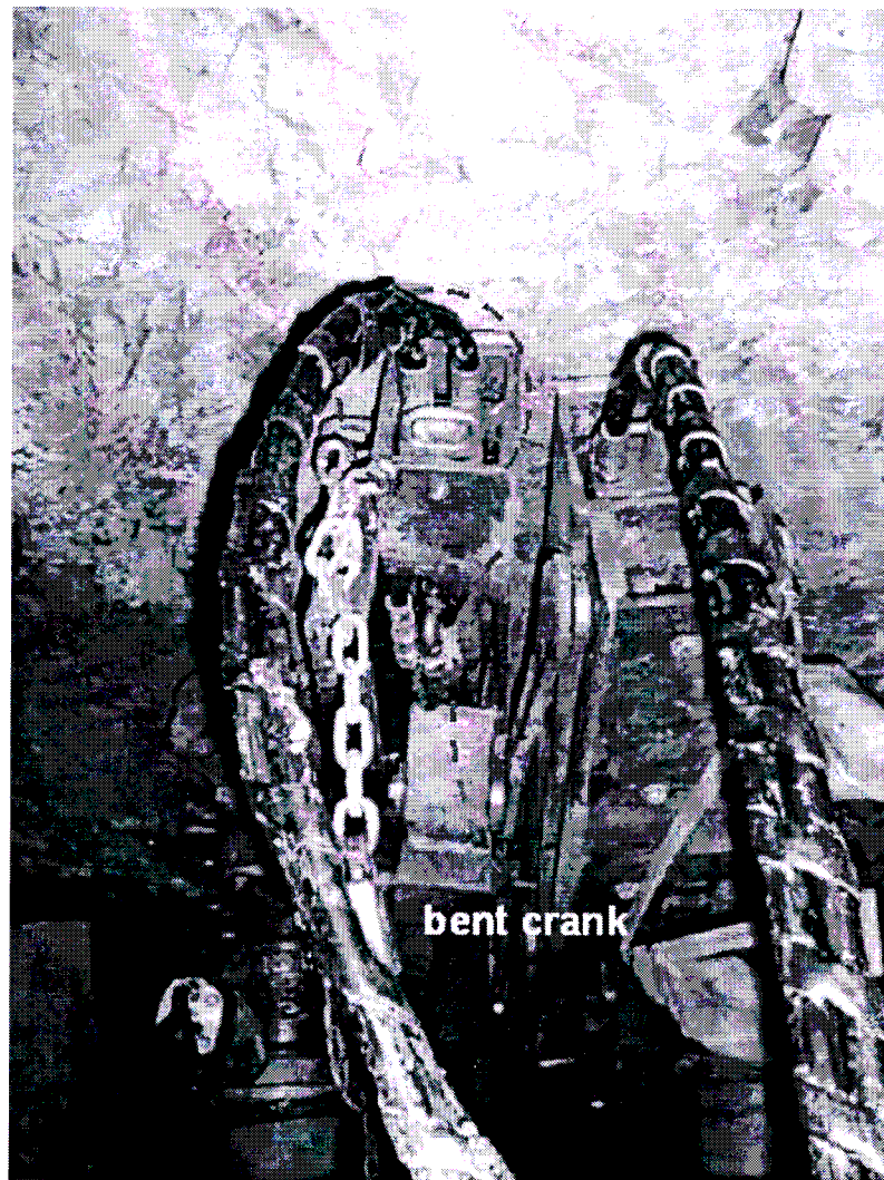
Figure 3-13 Underside of headboards showing the position of the hose adaptors at the back of the headboards, and the slightly deformed crank
