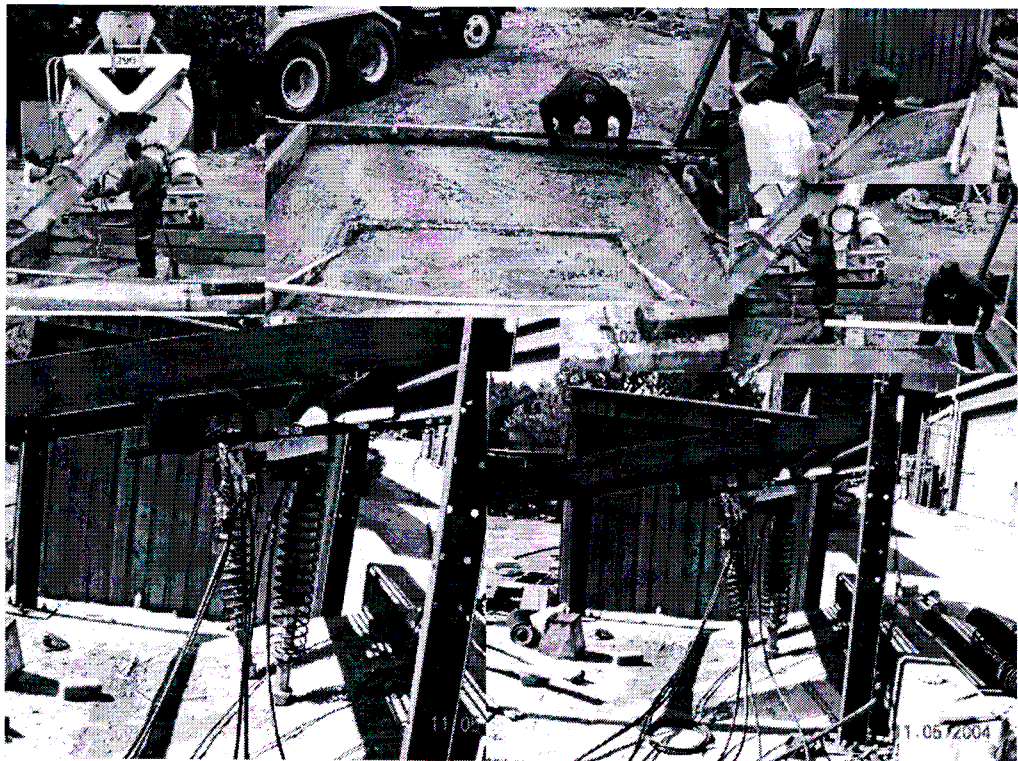
Figure 3-20 Collage of photos showing building of concrete foundation and testing of system in the rig
