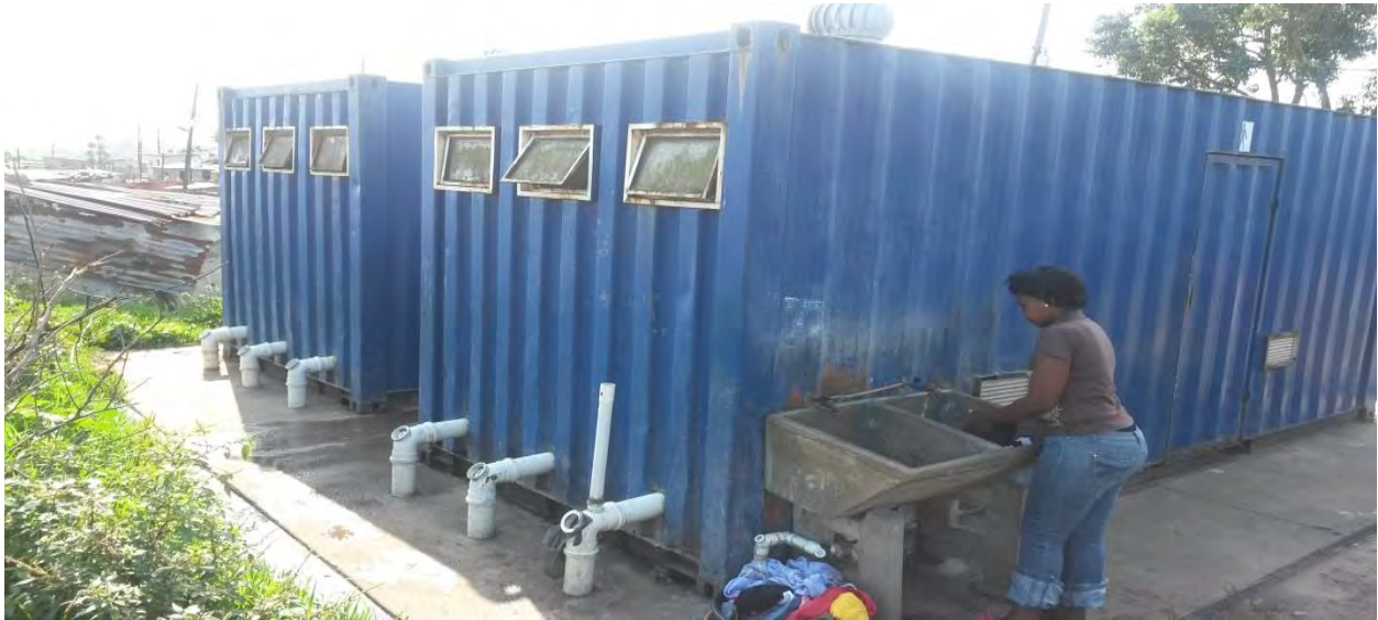
Figure 3: A containerized ablution facility in Magwaveni.
