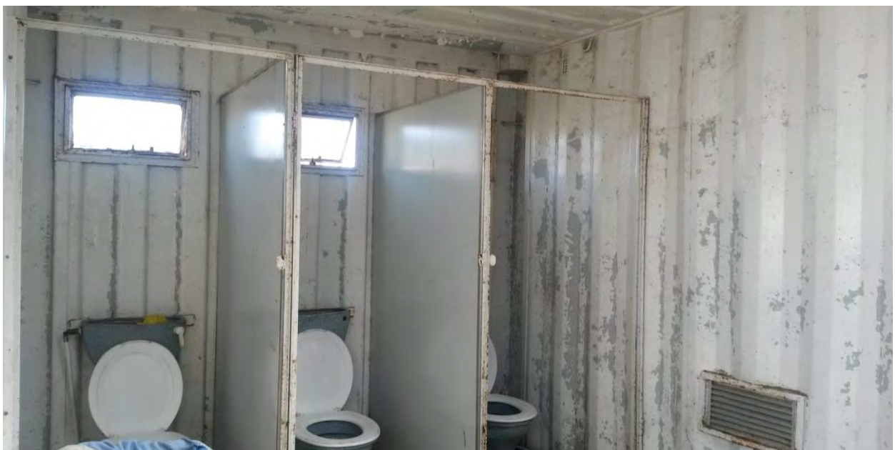
Figure 4: Flush toilets in a containerized ablution facility in Magwaveni.
